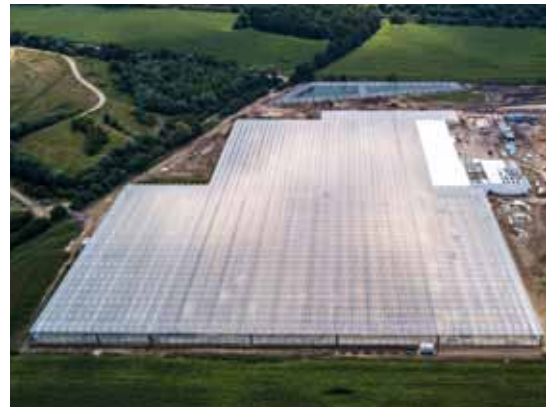
The greenhouse in Dolní Lutyně will be the largest production greenhouse in the Czech Republic with its area of 11 ha
