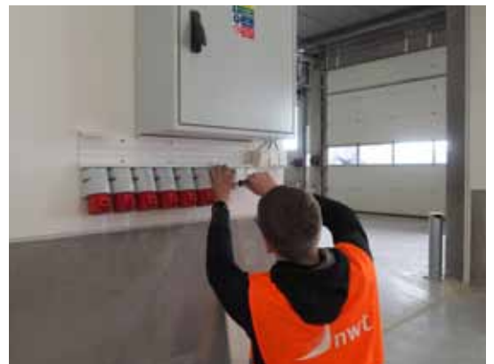
The Ptáček production hall in Olomouc has complete power installations, outdoor wiring and lighting
